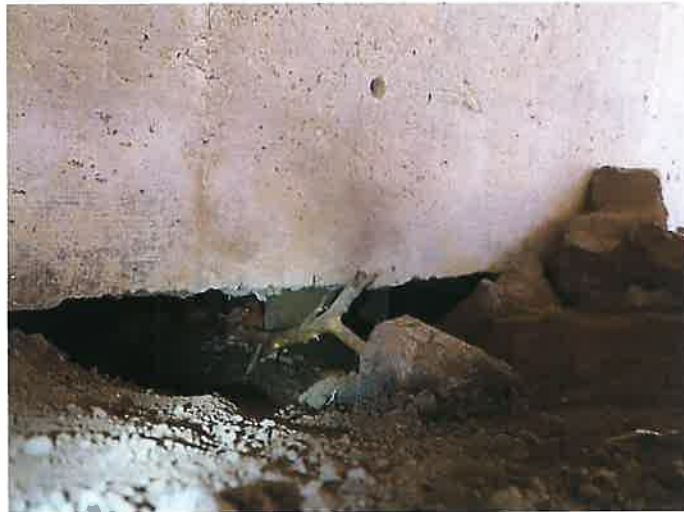
NORTH ABUTMENT UNDERMINED
