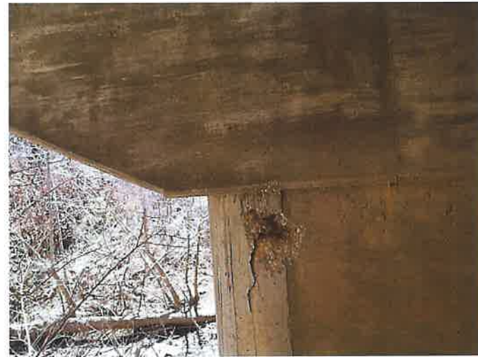
NORTH PIER, EAST END SPALL BELOW CAP
